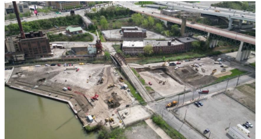
Pump station relocation and enabling infrastructure for Cavs/Clinic Global Peak Performance Center is already underway
